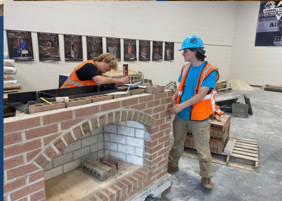
Masonry: Fireplaces & mailboxes
